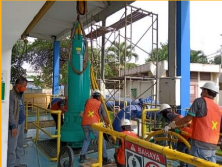
Installed Pump : - Water Distribution Pump
