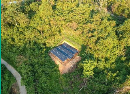
Installed Pump : - Solar Pump
