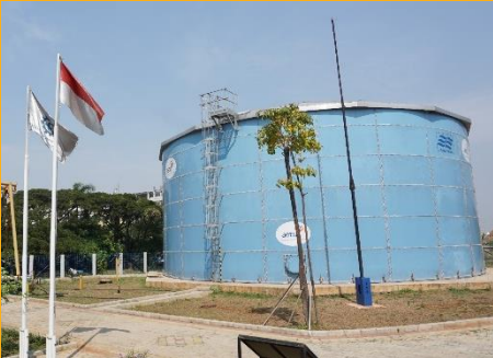
Installed Pump : - Booster Pump
