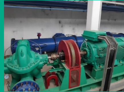
Installed Pump : - Water Distribution
