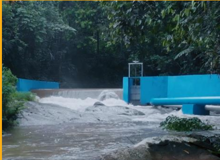
Installed Pump : - Water Distribution Pump
