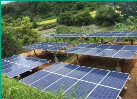
Installed Pump : - Solar Pump
